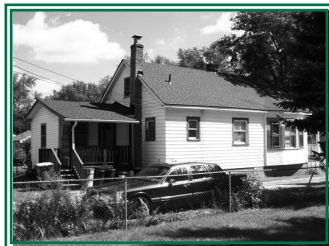
The owners of this house received a home repair loan to replace their roof through the Housing Rehabilitation Program.
